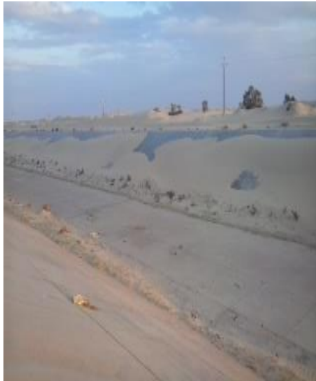
Figure 6. Sand accumulation in EL-Sheikh Gaber Canal at km 63.000.
